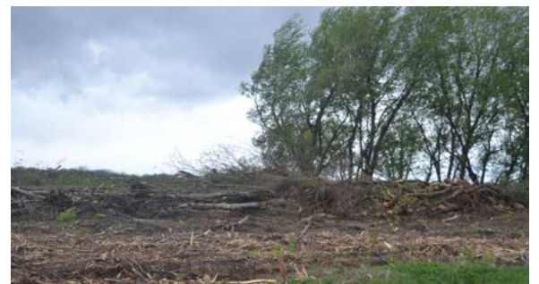
At the site of the future Mucci Greenhouses, a wooded area has to first be cleared. The downed trees and plant materials will be recycled into various types of mulches and soils as needed by the greenhouses.
